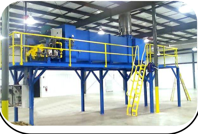
Below: S&B oxidizer installed at Bontex.
