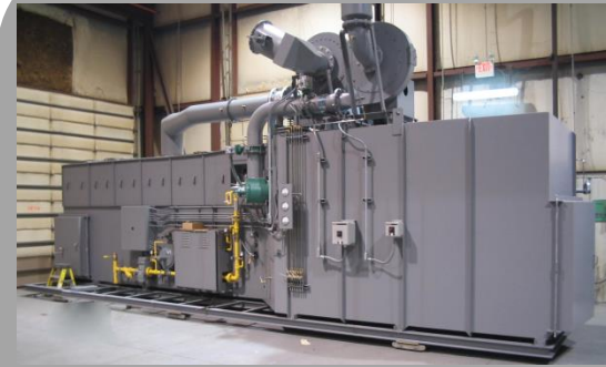
A Stelter & Brinck oxidizer installed at Western Digital
