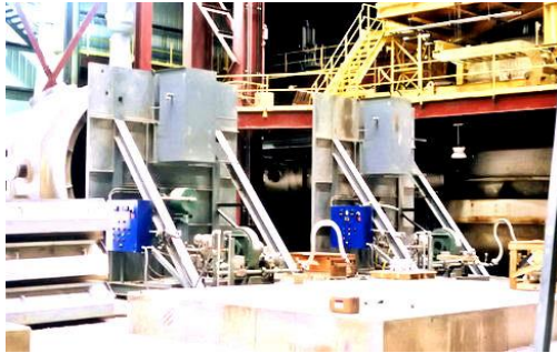
Ladle Dryers/ Dryer-Preheaters/ Preheaters
